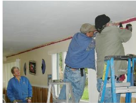
Quintin Mugas and Sal Salvino install the ceiling grids where the acoustic panels are glued and stapled. Charlie Romine looks on.
